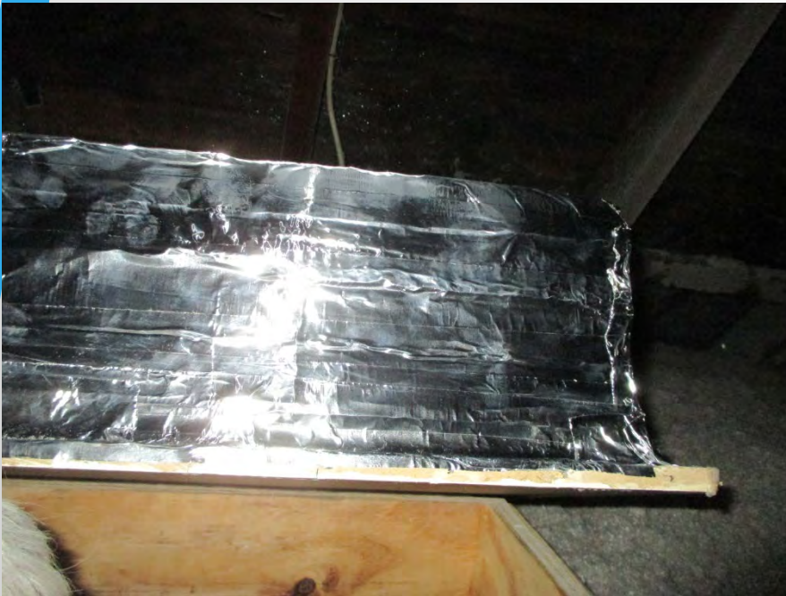
Insulated, sealed, and weatherstripped hatch cover
