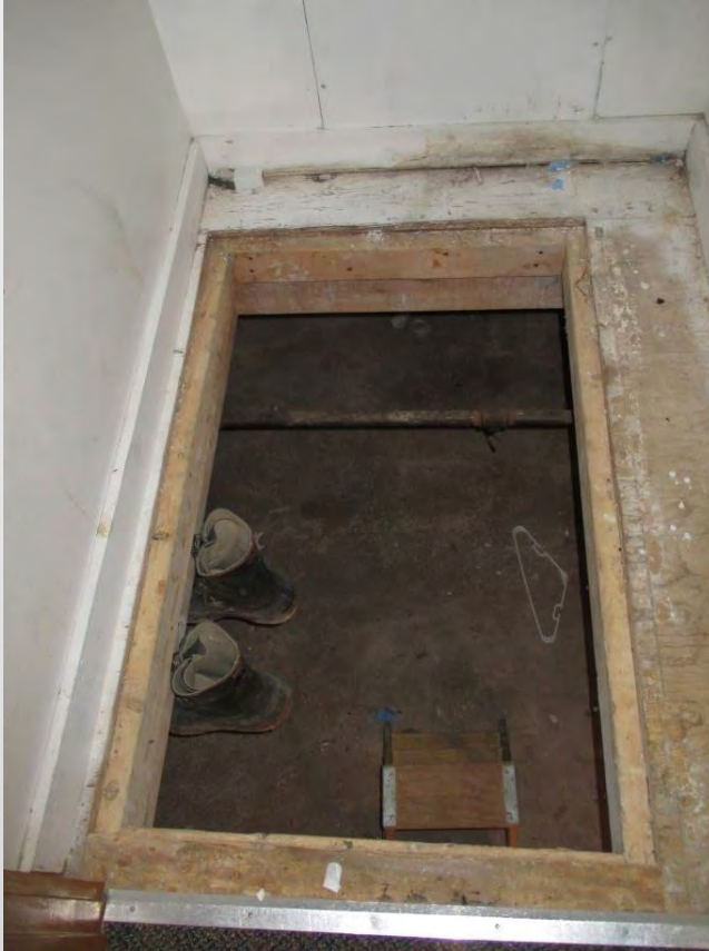
A crawlspace wet enough to warrant rubber boots
