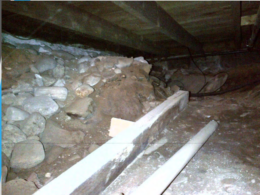
Impact to structure
