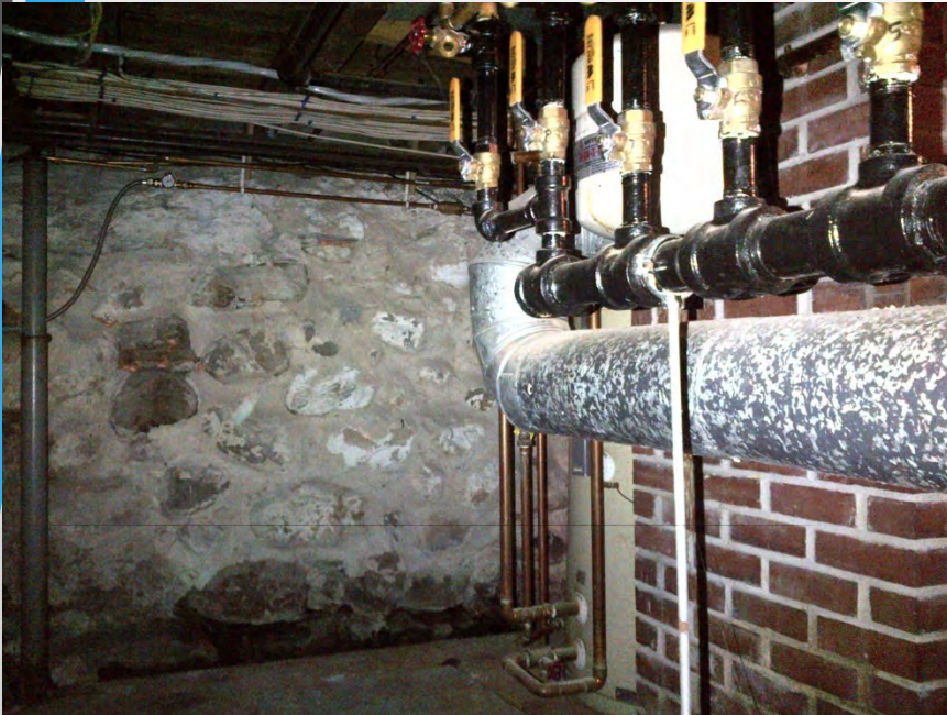
Seepage at base of foundation
