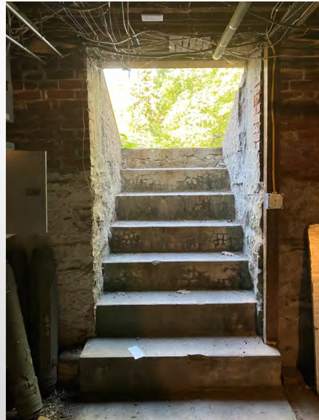
A wide open basement bulkhead entry
