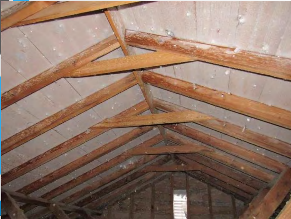
Green Building Advisor/Reuben Saltzman, Structure Tech
